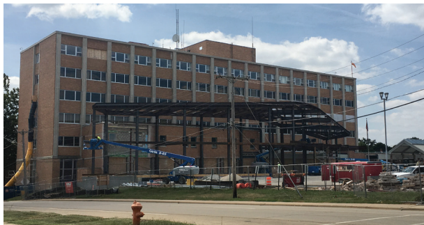
Construction at OSF HealthCare Center for Health – Streator is expected to be completed fall 2019.
